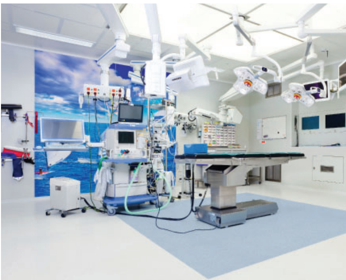
Sphera SD installed in an operating room
